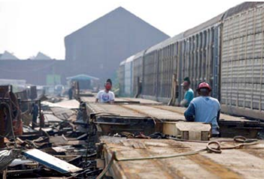
Dismantling railcars and recycling the waste is also a source of raw material for Mervis.
